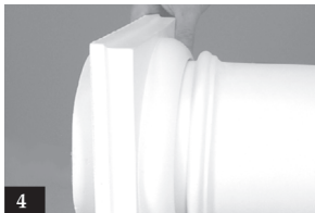
4. Slide the capital over the top of the column shaft allowing it to gently rest on the astragal.
