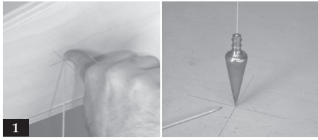
1. Drop a plumb bob from the center of the soffit to determine the column's center point on the floor. Mark this point for reference to align the shaft in the proper position.
