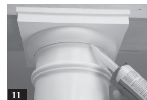
11. Apply a paintable silicone caulking between the capital and the shaft. (Note: Not all silicone caulking is paintable.)
